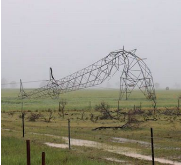
Cause of SA blackout: One of several collapsed electricity pylons near Melrose in South Australia's Mid North. (ABC News: Tom Fedorowytch)
